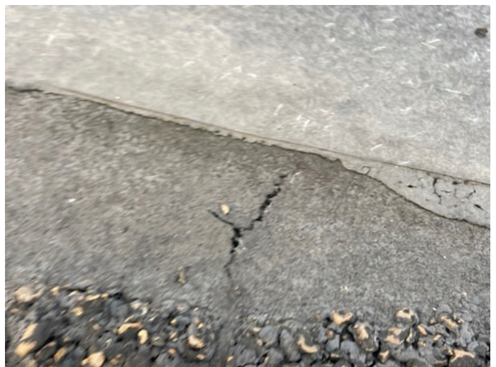
Cracks in membrane
