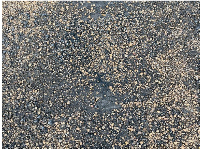
Cracks in membrane
