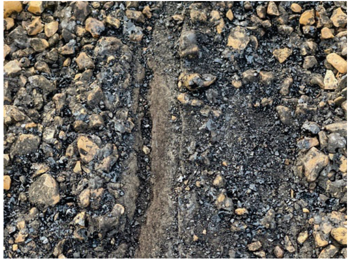
This crack is all the way through to the decking
