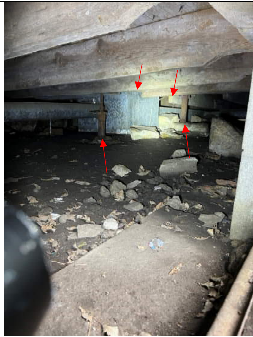
Photo 10: Jack posts, unsupported joists from an alternative angle, and a cut joist
