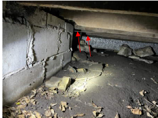
Photo 8: Unsupported floor joists ends
