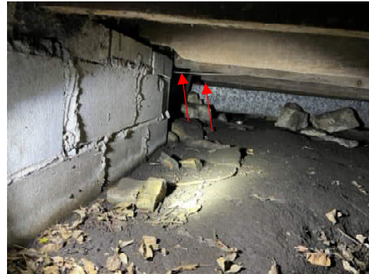
Photo 8: Unsupported floor joists ends
