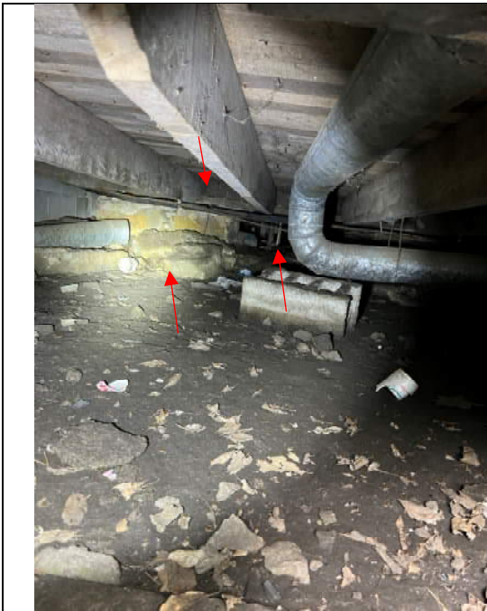
Photo 9: Southeast wing framing. Note the flush beam, stone remnants, and jack post
