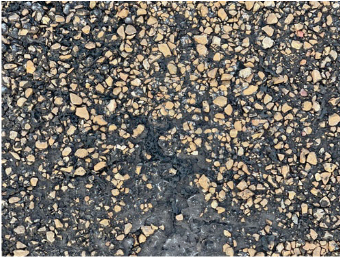
Cracks in membrane
