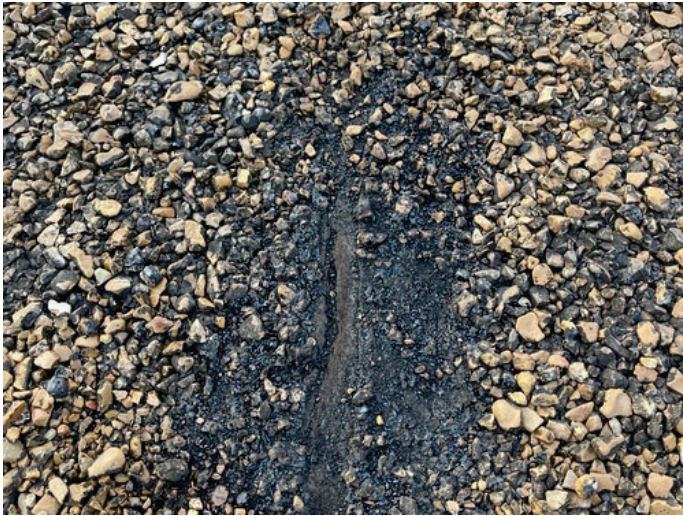
Cracks in membrane
