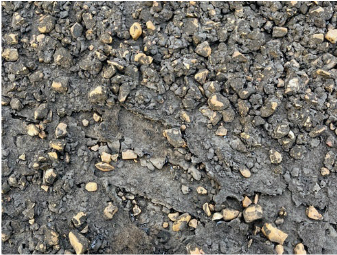
Cracks in membrane
