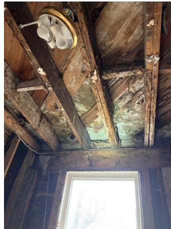
Image: 28: North addition framing deterioration
