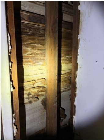
Image: 25: North addition framing deterioration
