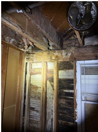
Image: 21: North addition framing deterioration
