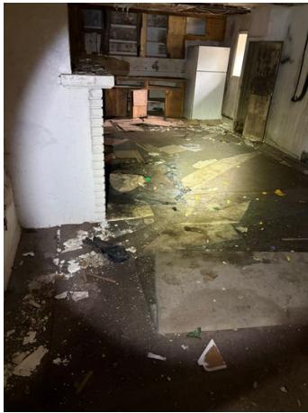
Image: 37: Debris covered floors
