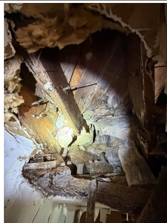
Image: 30: North addition framing deterioration
