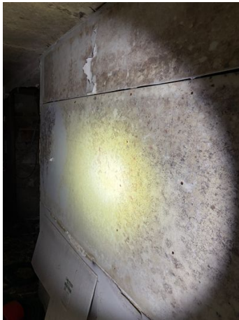
Image: 33: Mold covered wall finishes
