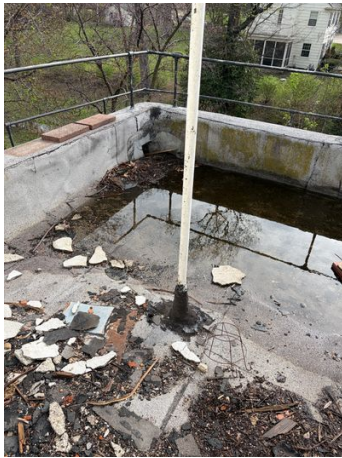
Image: 31: North addition roof ponding
