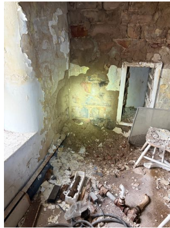
Image: 38: Debris covered floors
