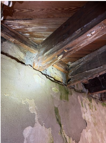
Image: 27: North addition framing deterioration
