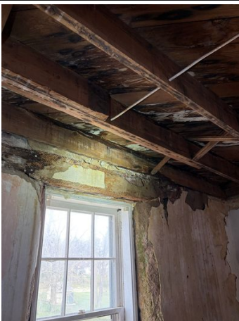
Image: 29: North addition framing deterioration
