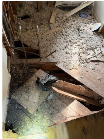
Image: 32: Missing floor sheathing
