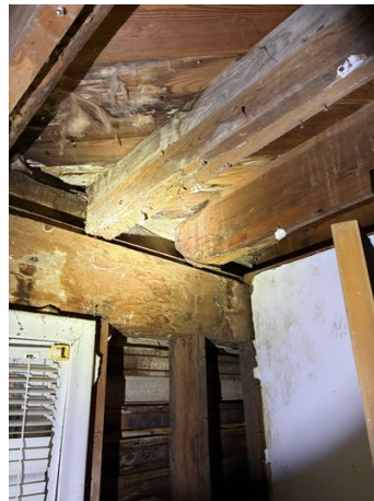
Image: 22: North addition framing deterioration
