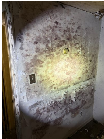
Image: 34: Mold covered wall finishes
