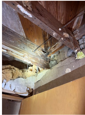
Image: 26: North addition framing deterioration
