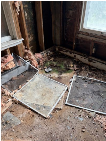
Image: 39: Debris covered floors
