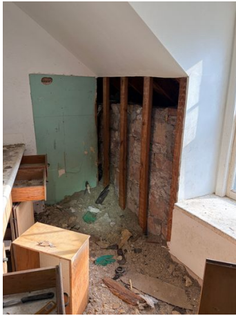
Image: 3: Deterioration at the southeast corner of the roof
