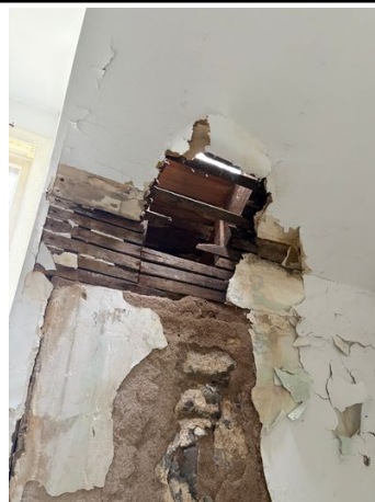
Image: 6: Deterioration at the northwest corner of the roof
