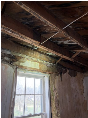
Image: 11: Floor framing deterioration below identified roof openings
