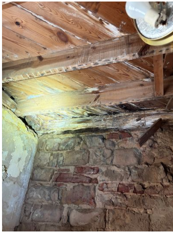
Image: 13: Floor framing deterioration below identified roof openings
