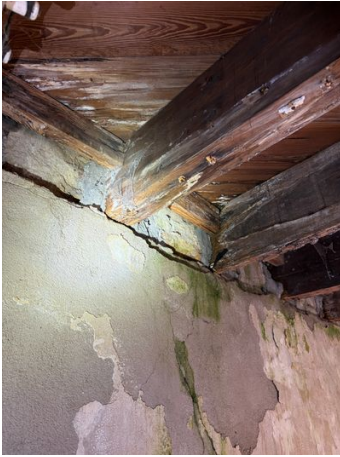
Image: 27: North addition framing deterioration
