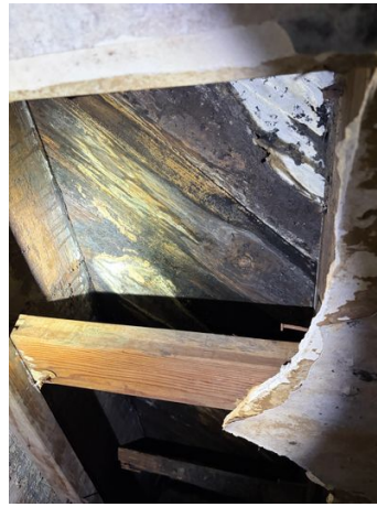
Image: 20: Floor framing deterioration below identified roof openings
