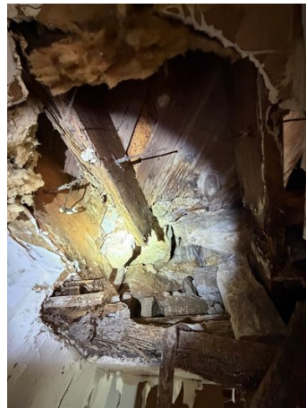
Image: 30: North addition framing deterioration
