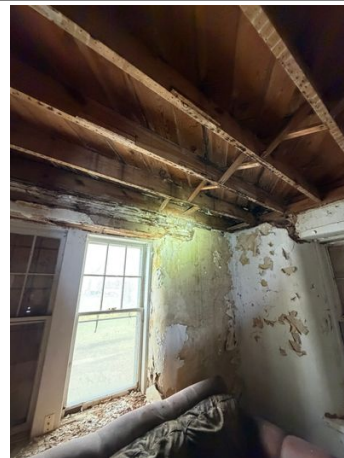
Image: 18: Floor framing deterioration below identified roof openings
