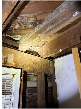
Image: 22: North addition framing deterioration
