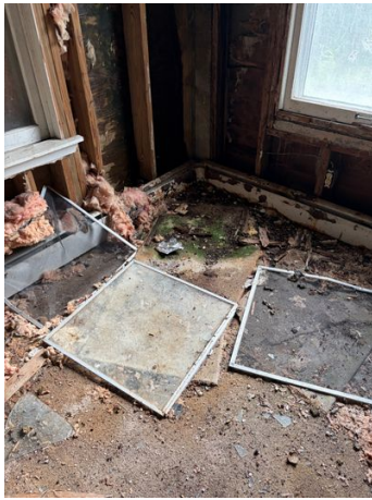
Image: 39: Debris covered floors
