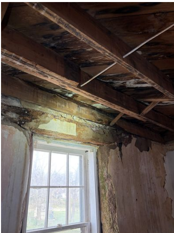
Image: 29: North addition framing deterioration
