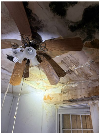
Image: 17: Floor framing deterioration below identified roof openings
