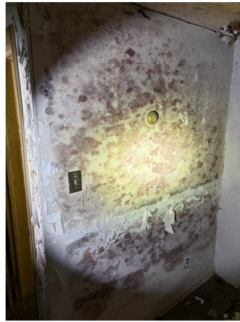
Image: 34: Mold covered wall finishes
