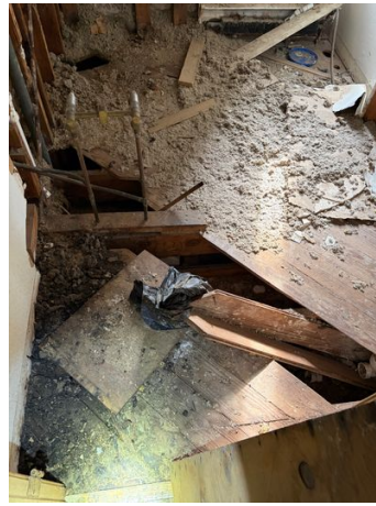
Image: 32: Missing floor sheathing
