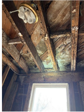
Image: 28: North addition framing deterioration
