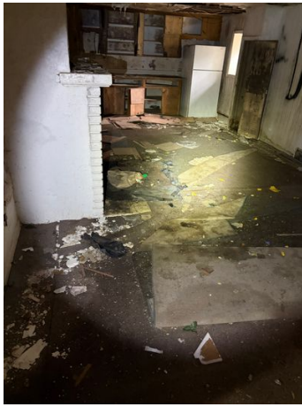
Image: 37: Debris covered floors
