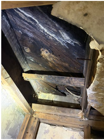
Image: 19: Floor framing deterioration below identified roof openings
