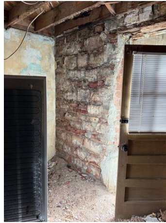
Image: 10: Floor framing deterioration below identified roof openings
