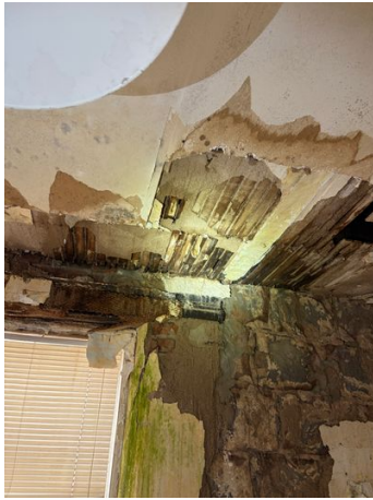
Image: 9: Floor framing deterioration below identified roof openings
