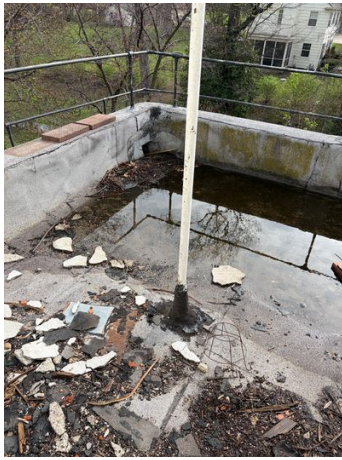
Image: 31: North addition roof ponding
