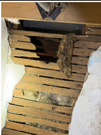
Image: 5: Deterioration at the southeast corner of the roof
