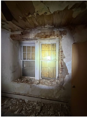
Image: 15: Floor framing deterioration below identified roof openings
