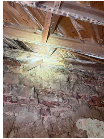
Image: 14: Floor framing deterioration below identified roof openings
