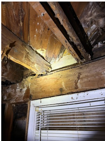
Image: 23: North addition framing deterioration
