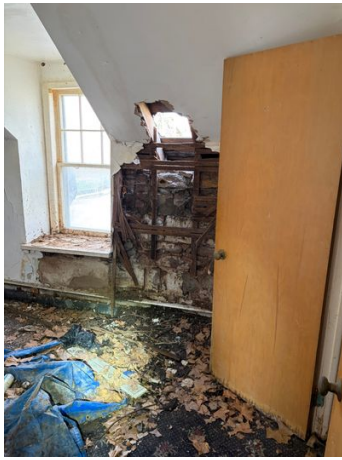
Image: 1: Deterioration at the southwest corner of the roof
