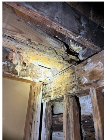
Image: 24: North addition framing deterioration
