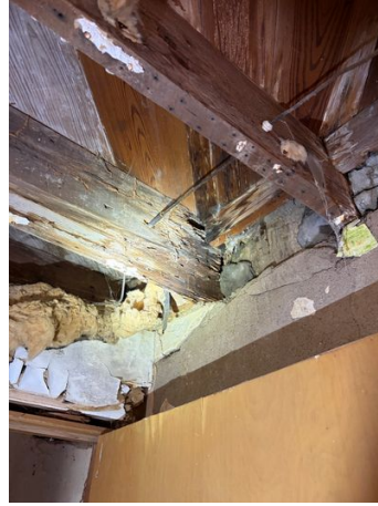
Image: 26: North addition framing deterioration
