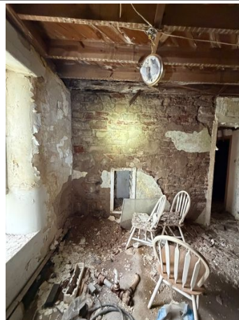
Image: 12: Floor framing deterioration below identified roof openings
