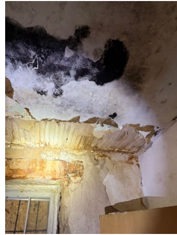
Image: 16: Floor framing deterioration below identified roof openings
