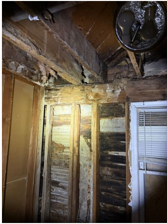
Image: 21: North addition framing deterioration
