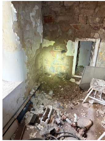
Image: 38: Debris covered floors
