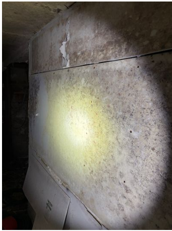
Image: 33: Mold covered wall finishes
