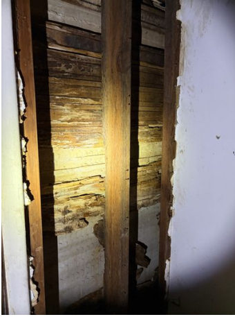
Image: 25: North addition framing deterioration
