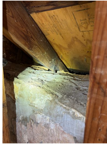
Image: 4: Deterioration at the southeast corner of the roof
