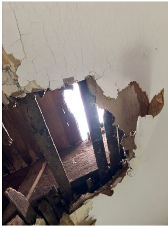
Image: 7: Deterioration at the northwest corner of the roof
