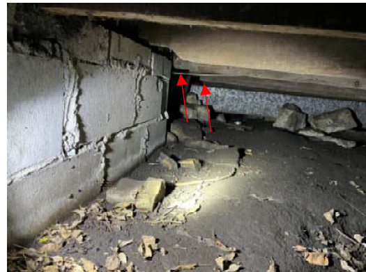
Photo 8: Unsupported floor joists ends
