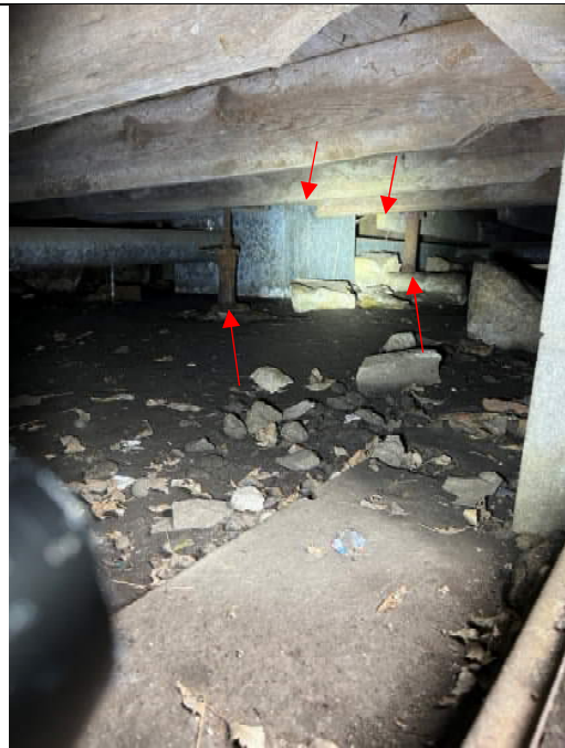
Photo 10: Jack posts, unsupported joists from an alternative angle, and a cut joist
